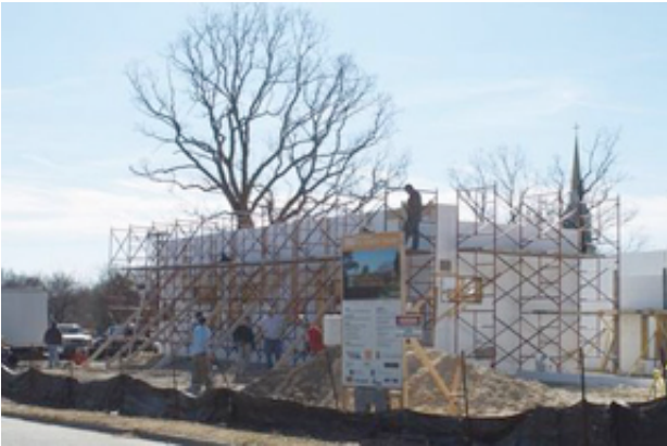
my sister's house taking shape. photo courtesy of the urban studio blog.
